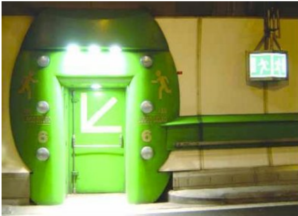
Figure 13: Examples from the Mont Blanc Tunnel: tunnel escape route and tunnel escape route sign.
